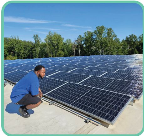
Saunders with the solar panels on the roof of The Center.
